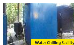
Water Chilling Facility
